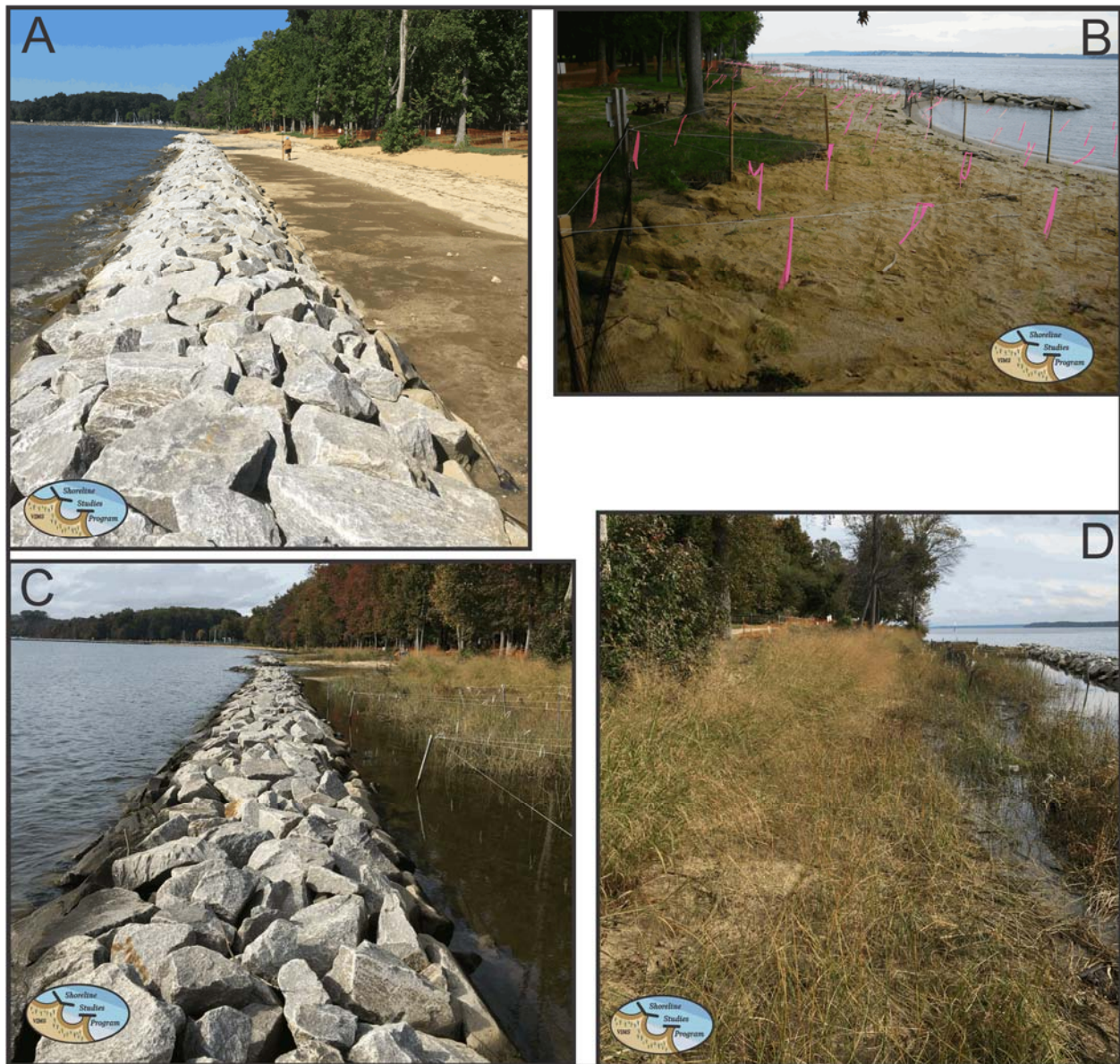
Figure 5. A) Rock sill 1 and sand fill after installation but before marsh planting (12Aug2016); B) Marsh grass planting and goose fence installation (1Sep2016); C) Sill 1 approximately one year after installation (23Oct2017); and D) high marsh grasses behind sill 1 after about one year (23Oct2017). Photos by Shoreline Studies Program, VIMS.
