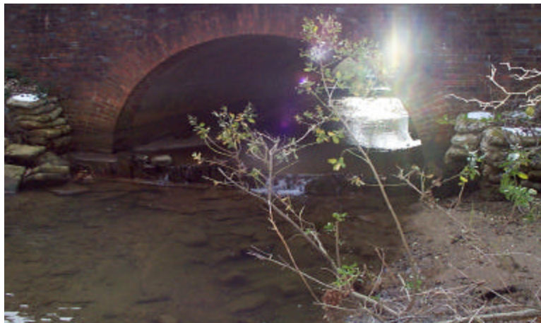
Figure 2. Brackens Pond spillway and tailrace. Irish ramp was set against the right wall on upstream end of culvert.
